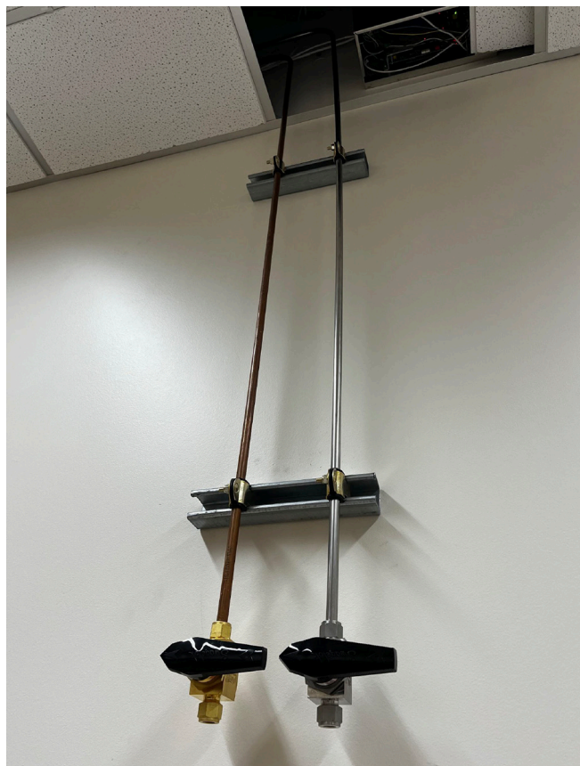
Figure 2: Compressed Air (left) and House Nitrogen Gas Lines Ran in Lab 238. We installed six of these valves and their pipework under Paul's supervision.
