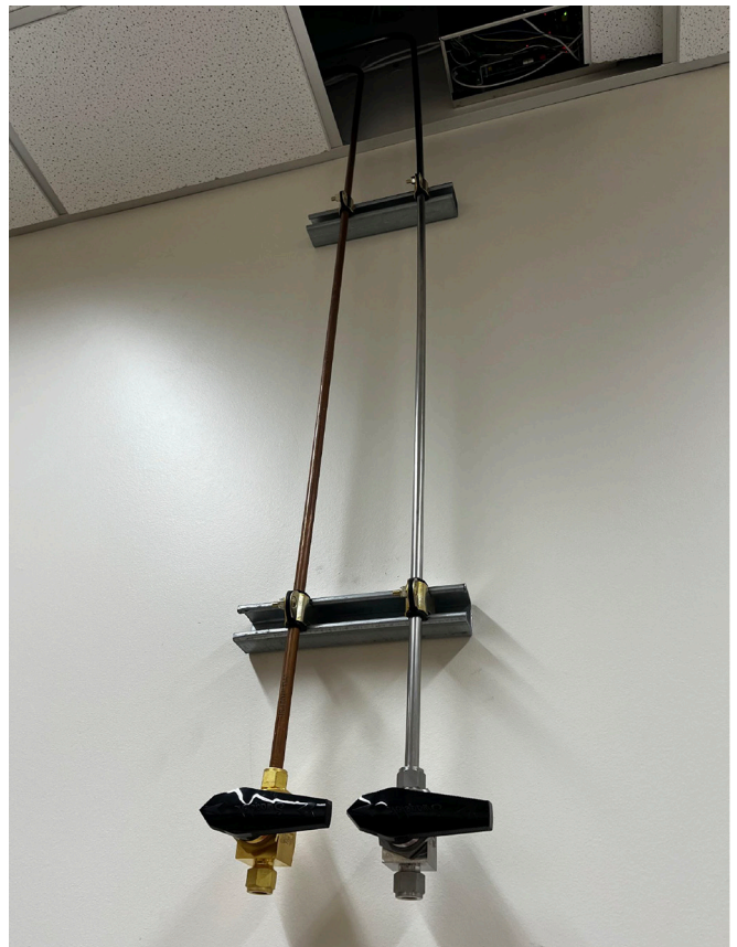
Figure 2: Compressed Air (left) and House Nitrogen Gas Lines Ran in Lab 238. We installed six of these valves and their pipework under Paul's supervision.
